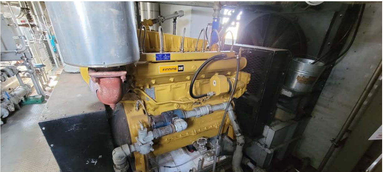
Engine was replaced on warranty and is stored in mineral oil.
