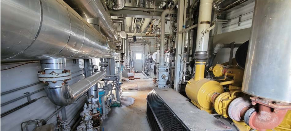
CAT 3306TA (203HP) Engine driving Mycom Reciprocating Compressor – Fuel gas can be utilized from 2 skid connections; at the outlet of the gas/gas exchanger, or pipeline gas
