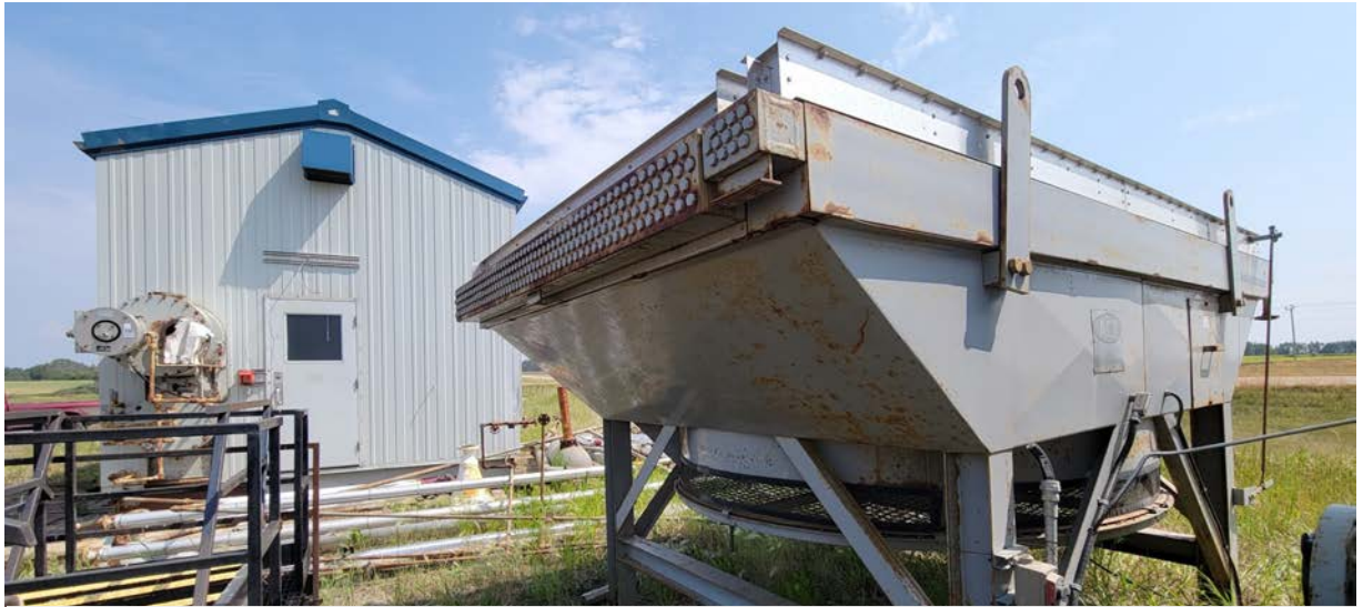
Condensate fin tube cooler for cooling hydrocarbon liquid from the tower before being sent for condensate storage
