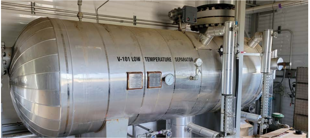
Low Temp Separator and plenty of boxed spare parts and consumables
