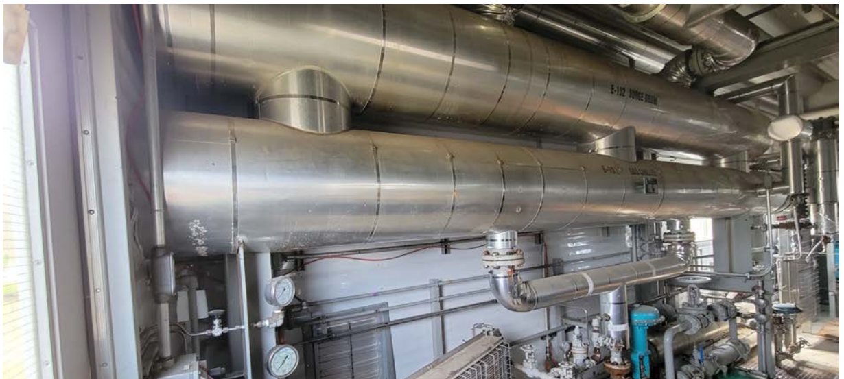
1.9MMBTU/Hr 1440psig Gas/Gas Exchanger
