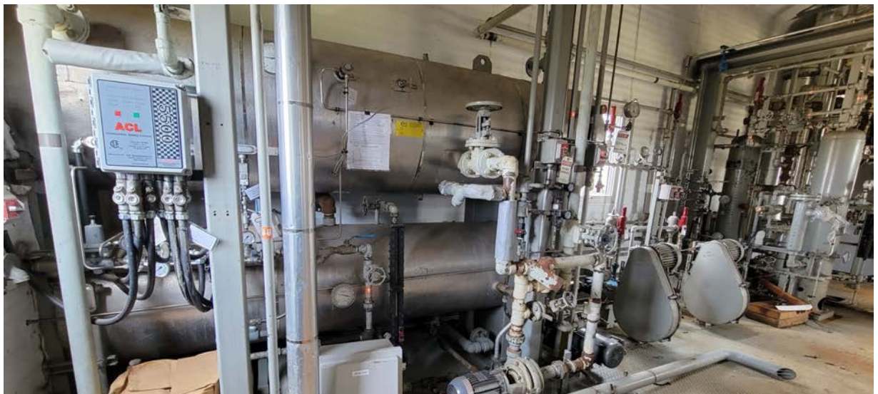
500,000BTU/Hr Glycol Regeneration system c/w ACL 5100 CSA Approved Burner Management System
