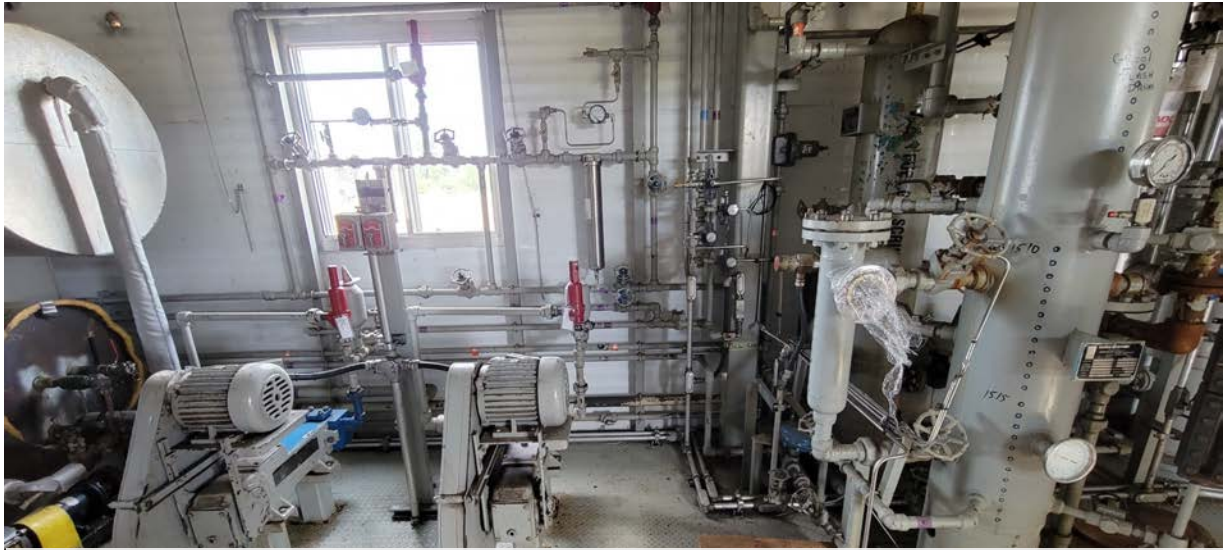
Duplex positive displacement pumps c/w HOA's as part of a comprehensive electrical package
